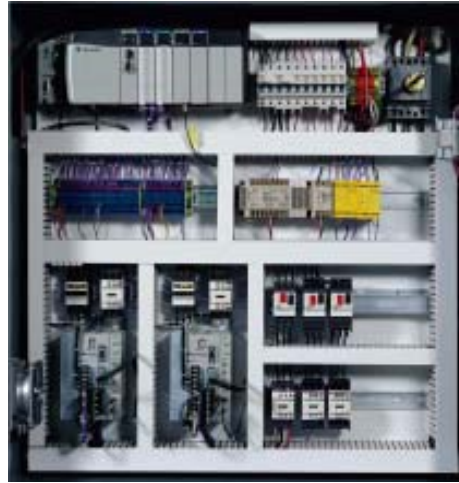
Allen Bradley PLC
